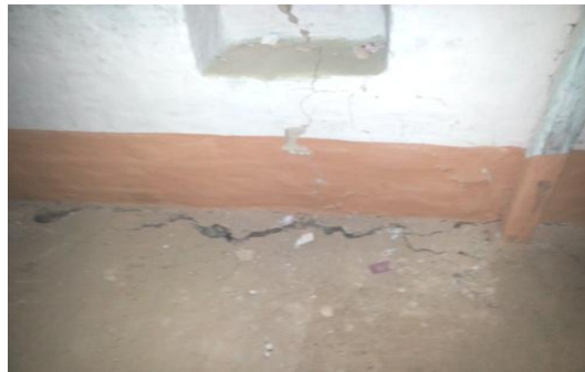
Cracked home of Subina Bishwokarma
