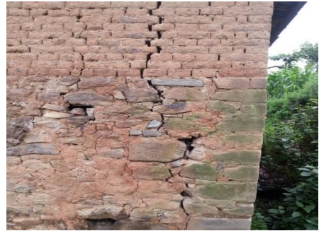
Cracked house of Anchali Lama
